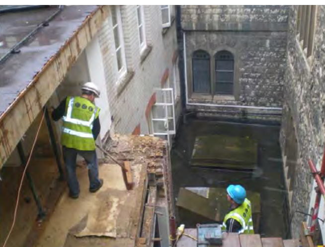
The removal of three stories of the former Museum building to create the new Link Gallery, 2009 (below).
